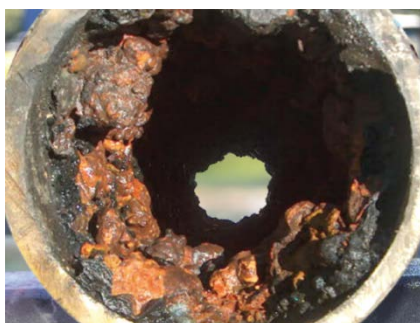
Typical Cast Iron Pipe Tuberculation
