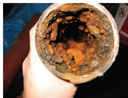
Typical Galvanized Steel Pipe Corrosion
