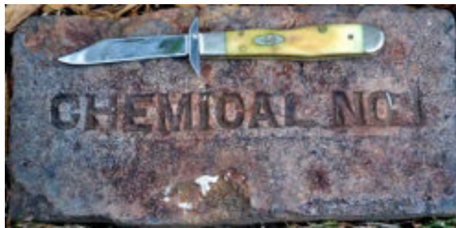
Figure 30: A treated foundation brick typical of many of those used in brick piers
