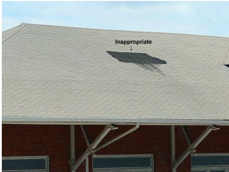
Figure 143: Chimney and smokestack removal is not appropriate
