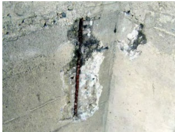
Figure 159: Iron-jacking is a common result of moisture problems in historic concrete
