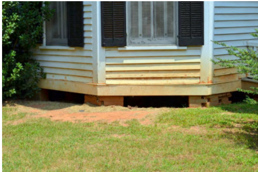
Figure 28: One of the few unfilled pier foundations in the Residential Sub-District
