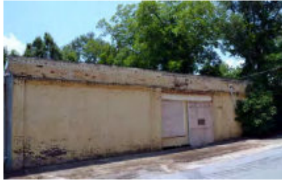
Figure 123: One of the earlier warehouses in the Industrial Sub-District Notice the ornamented nature of this nineteenth century example.
