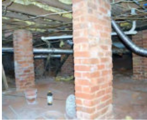
Figure 29: A brick pier foundation under a historic home in the Residential Sub-District
