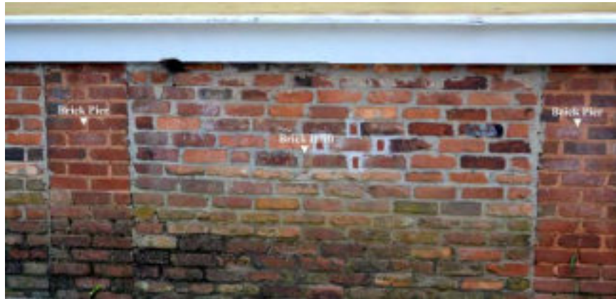
Figure 31: An example of brick infill in a brick pier foundation in the Residential Sub-District
