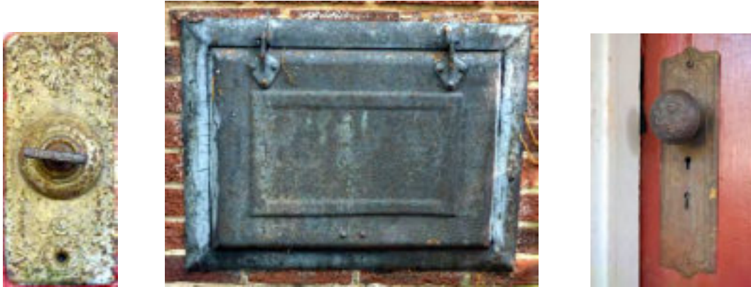
Historic doorbell (left), historic coal chute (middle), historic door hardware (right) Figure 53: Some examples of miscellaneous elements of significance
