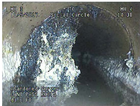
Impassable Root Intrusion with Grease Build-Up at Paige Court
