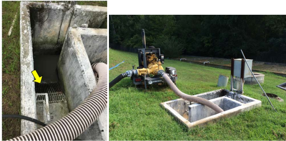
Figure 13 - Raw Sewage Pumping Station
