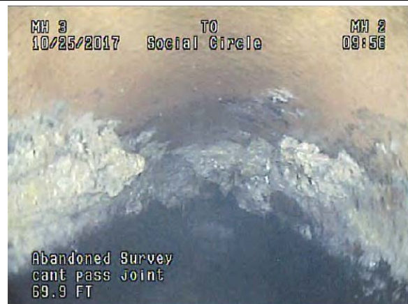
Impassable, Separated Joint with Grease Build-Up in Clay Pipe on Fairplay Drive
