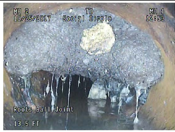
Root Intrusion in Clay Pipe on North Cherokee
