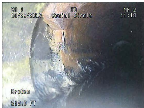
Broken Pipe at Material Change of Pipe on Ronthor Drive
