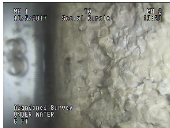
Camera Underwater and Grease Deposits at Memorial Street Creek Crossing
