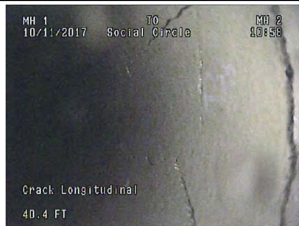
Crack in Clay Pipe at Paige Court
