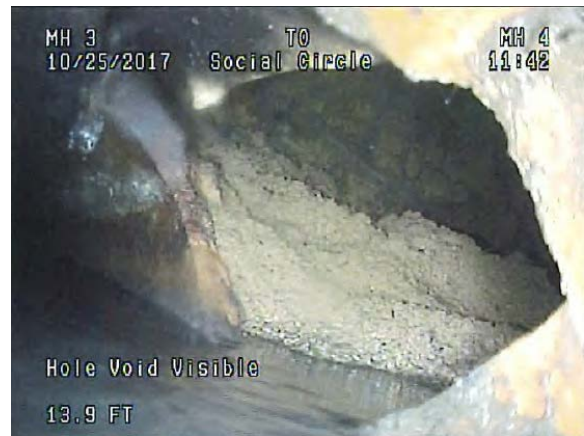
Hole in Clay Pipe on Ronthor Drive
