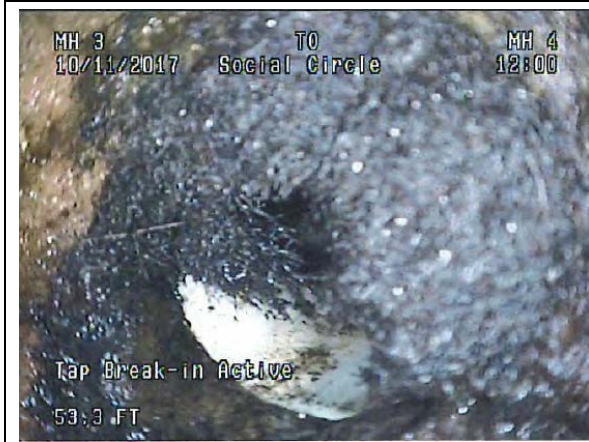
Root Intrusion at a Tap in Clay Pipe at Marco Estates
