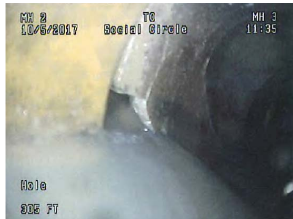
Hole in Clay Pipe at West Hightower Trail
