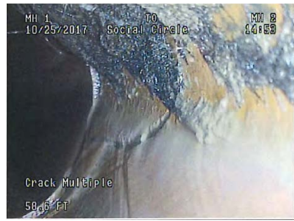
Cracks and Roots in Clay Sewer at Carvar Drive Wetwell
