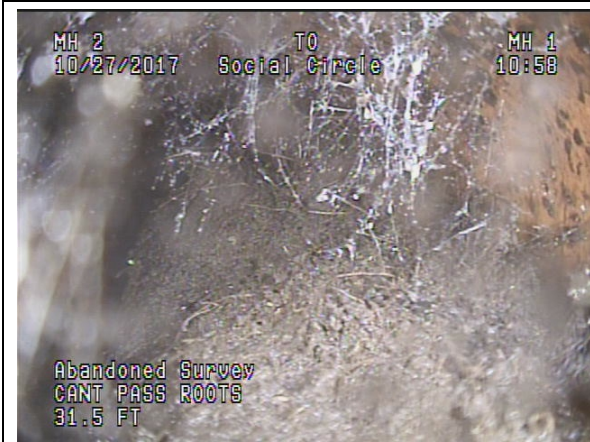
Root Intrusion in Clay Sewer Pipe South Cherokee Road Outfall
