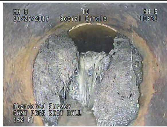
Root Intrusion in Clay Sewer Pipe Hickory Drive
