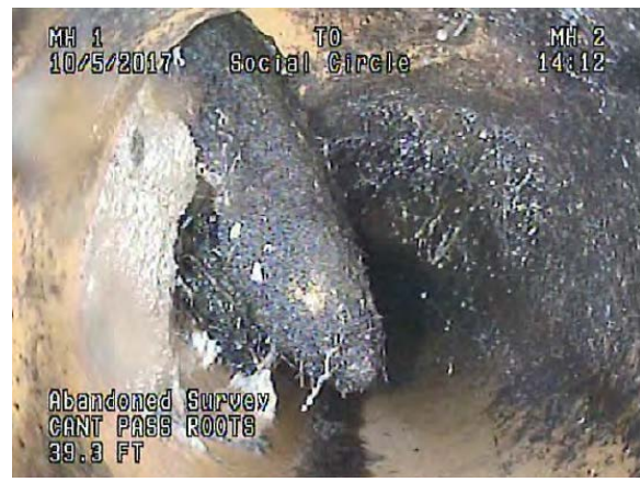
Impassable Root Intrusion at a Tap on Paige Court
