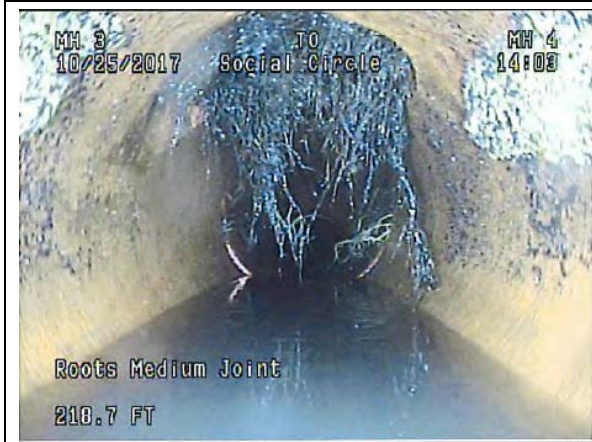
Root Intrusion at a Tap in Clay Pipe on North Cherokee
