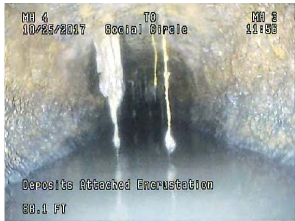
Encrustation in Clay Pipe on Ronthor Drive
