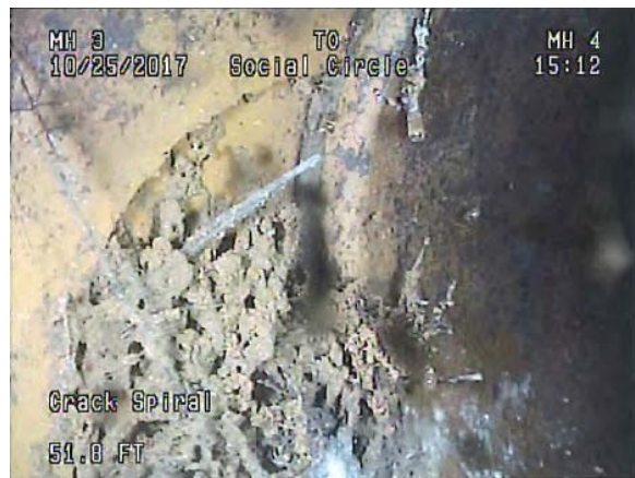
Spiral Crack in Clay Sewer at Carvar Drive Wetwell
